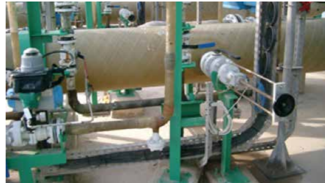
GRF- pipe of a seawater desalination plant
