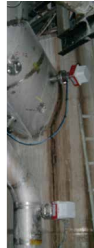
Installation after completion in cooling circuit of the “Three Gorges hydro-electric dam” (China)
